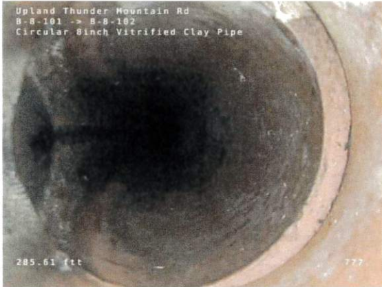
1_6_2025 9_43_05 AM_e895b841-ed7d-4bb8-a67f-98cb8eaa94e8_20250106_10 2033_012.jpg, 00:31:30, 285.61ft Tap Saddle Activity at 9 o'clock, dia/height: 4inch
