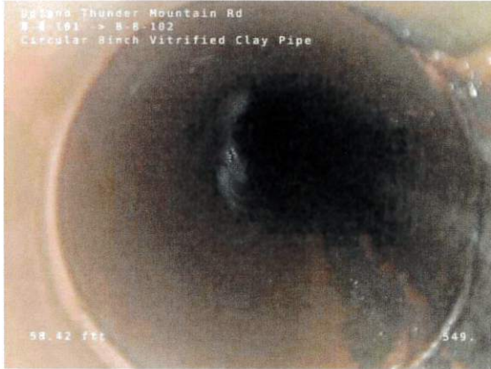
1_6_2025 9_43_05 AM_6663fc2c-66ab-4112-a087-b81566e594fc_20250106_094 941_378.jpg, 00:02:03, 58.42ft Tap Saddle Activity at 3 o'clock, dia/height: 4inch
